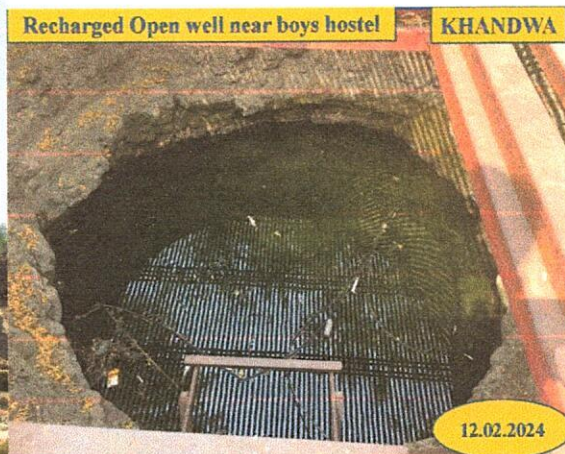
Recharged open well near boys hostel
