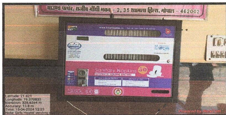
Installation of sanitary napkins vending machines in girls hostel
